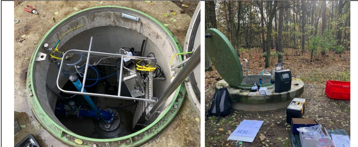
Figure 2 Flow cytometer installed in well chamber (left); flow cytometer maintenance and manual measurements (right) (©Christoph Sprenger)
